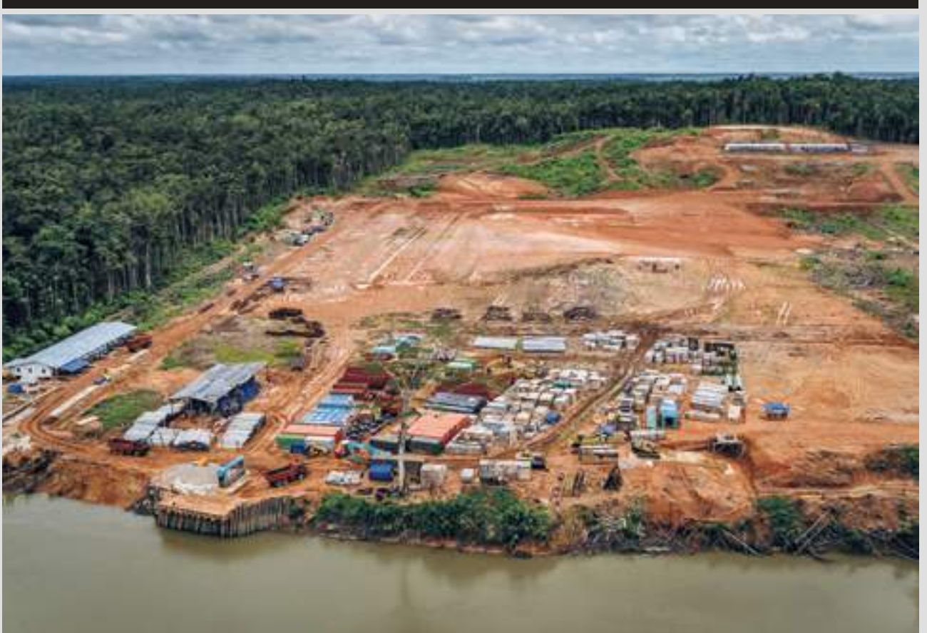
1 April 2018, PT Tulen Jayamas Timber Industries construction site in PT Kartika Cipta Pratama (HSA), Papua, 6°22'49.025"S 140°18'48.047"E ©Ifansasti/Greenpeace
